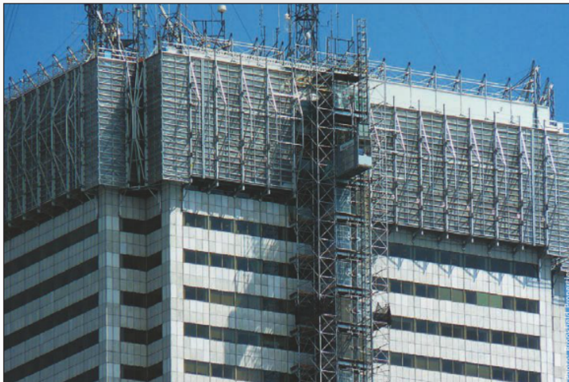
First Canadian Place, Toronto: $130 million retrofit and recladding of Canada's tallest office tower. The 45-year old, 72-storey, 2.8-million-square-foot building had the latest mechanical and electrical systems installed and marble façade replaced. Result: Annual energy saving cut by 17 per cent; increased leaseable space. Payback: 16 years.
